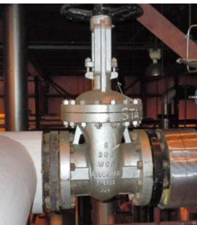
■ Non insulated valve
